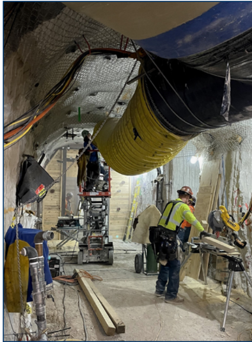
The crafts needed to complete the horizontal concrete plug included carpenters and ironworkers who built the bulkheads needed to support five separate grout pours over five months.
