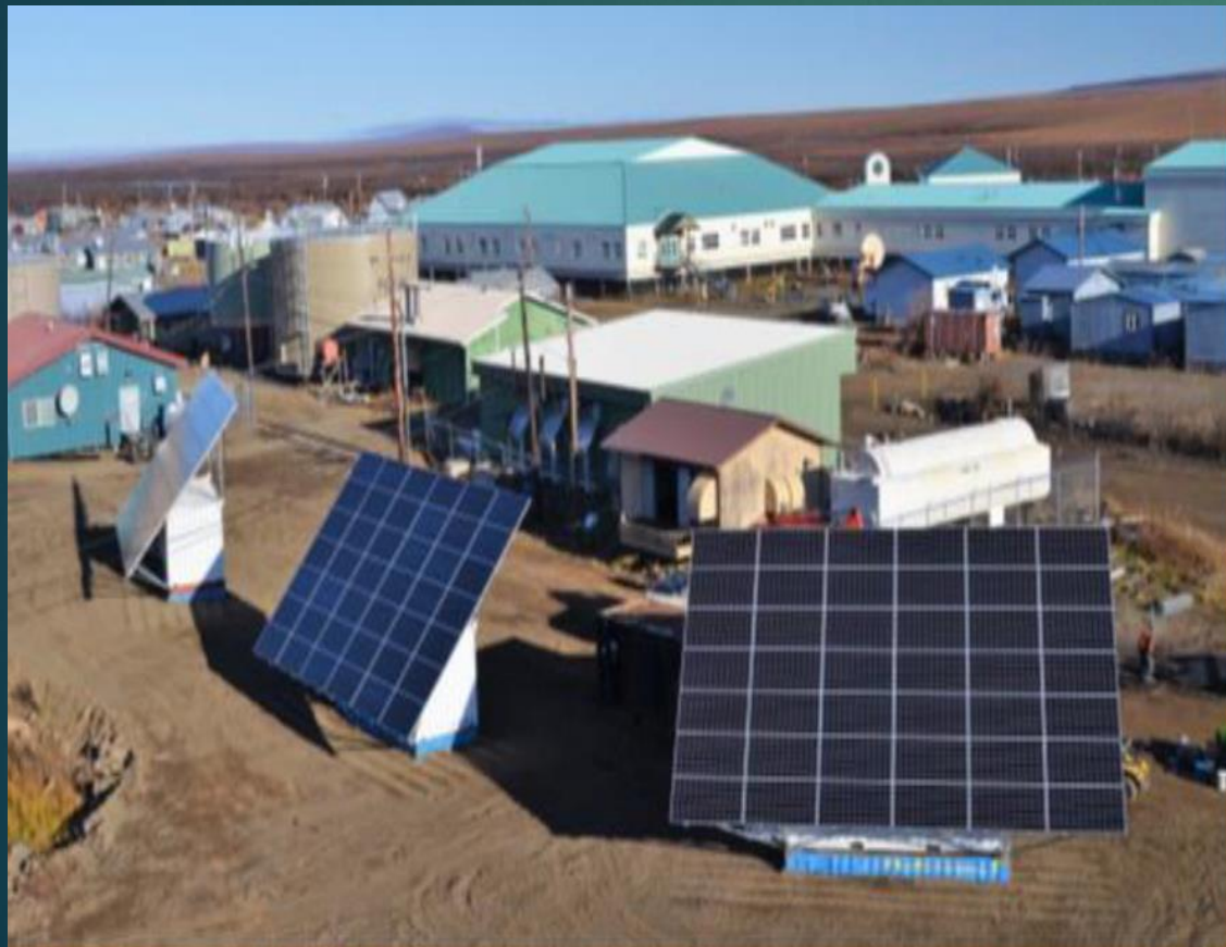
Buckland Solar arrays, Courtesy NANA
