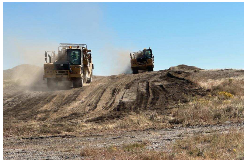
Excavators make progress on Cell 3, a new disposal cell at the ICDP.
