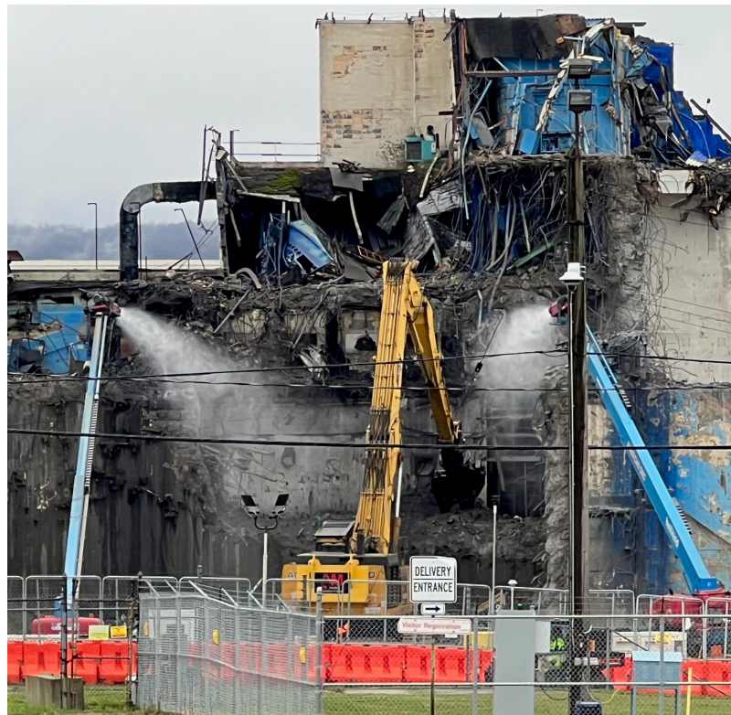
Main Plant Process Building deconstruction of the hot cells, which were used during spent fuel reprocessing operations.
