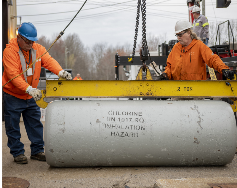
Paducah Site maintenance mechanics remove the last 1-ton chlorine cylinder from the C-611 Water Treatment Plant, a significant reduction of hazards at the site.
