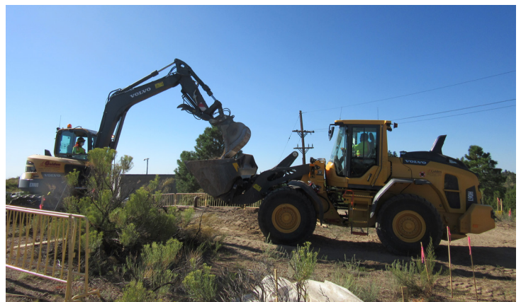
An excavation crew removes contaminated soil from legacy Los Alamos National Laboratory operations in North Ancho Canyon.
