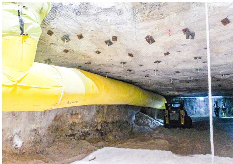
When Utility Shaft crews reached repository depth, horizontal excavation began to connect the shaft with the WIPP mine.
