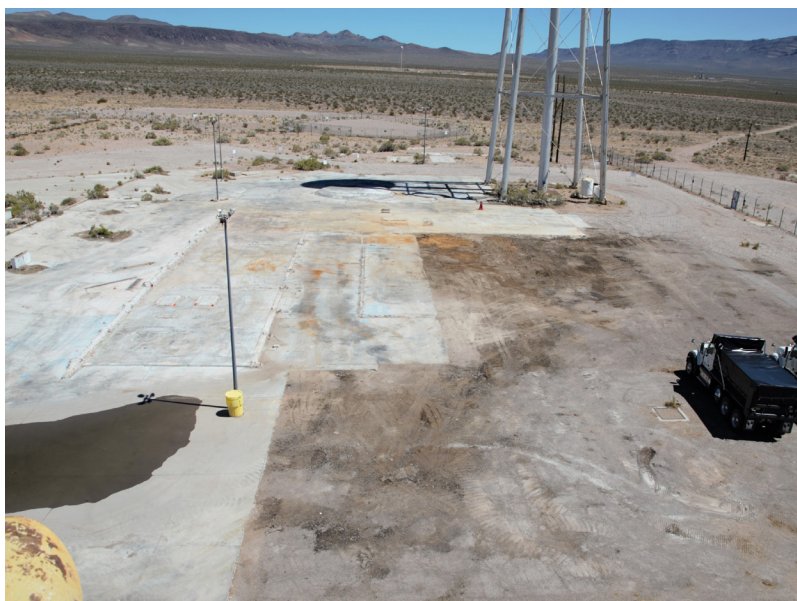
An aerial look at the demolition of ancillary structures at TCC early in the demolition work and following completion of the work.
