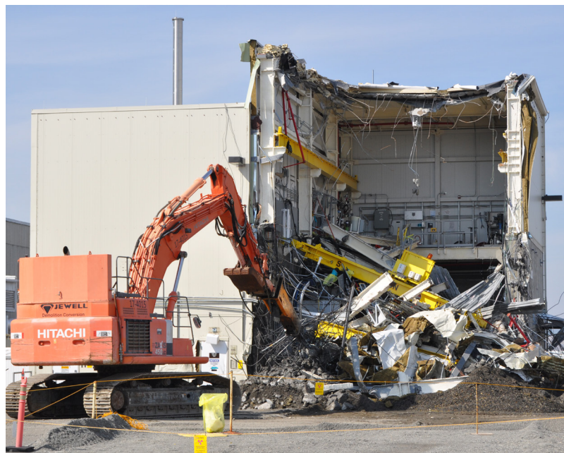
Hanford crews demolish the facility used to transfer radioactive sludge out of a nuclear fuel basin in the K West Reactor.
