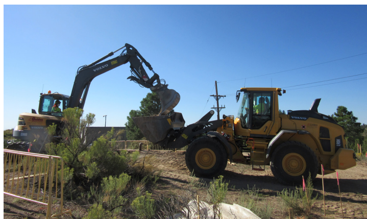
An excavation crew removes contaminated soil from legacy Los Alamos National Laboratory operations in North Ancho Canyon.
