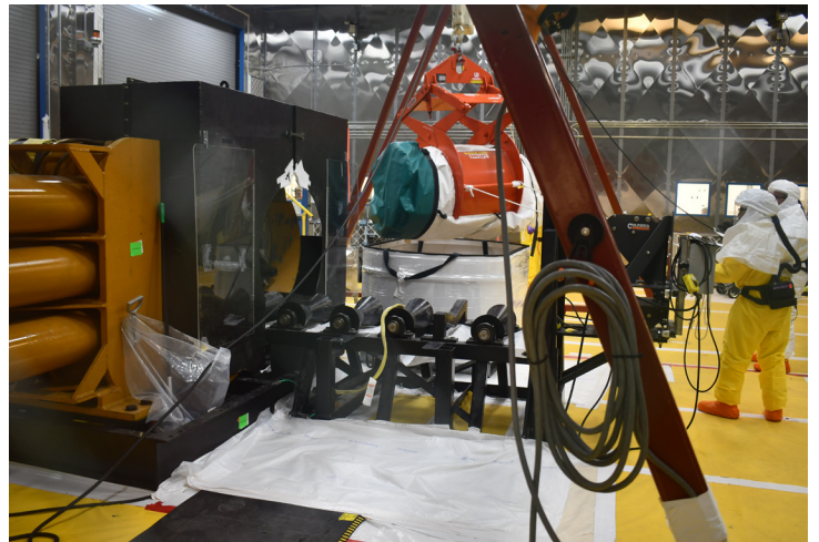
Waste Retrieval Operations crew guide a cut section of CMP filled with cemented TRU waste into a standard waste box in preparation for shipment and permanent disposal at WIPP.
