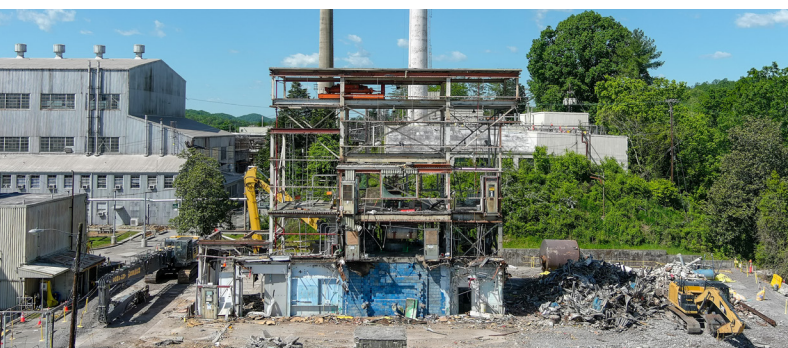
Crews safely take down the Low Intensity Test Reactor in ORNL's central campus.
