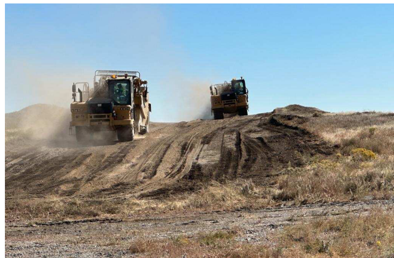
Excavators make progress on Cell 3, a new disposal cell at the ICDF.
