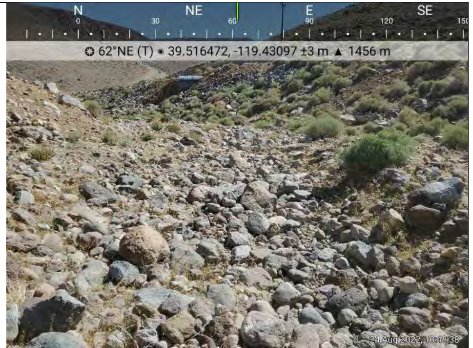
Photo 24. Looking downstream at AR 1, culvert coming in is the end of the relevant reach for the accompanying report.
