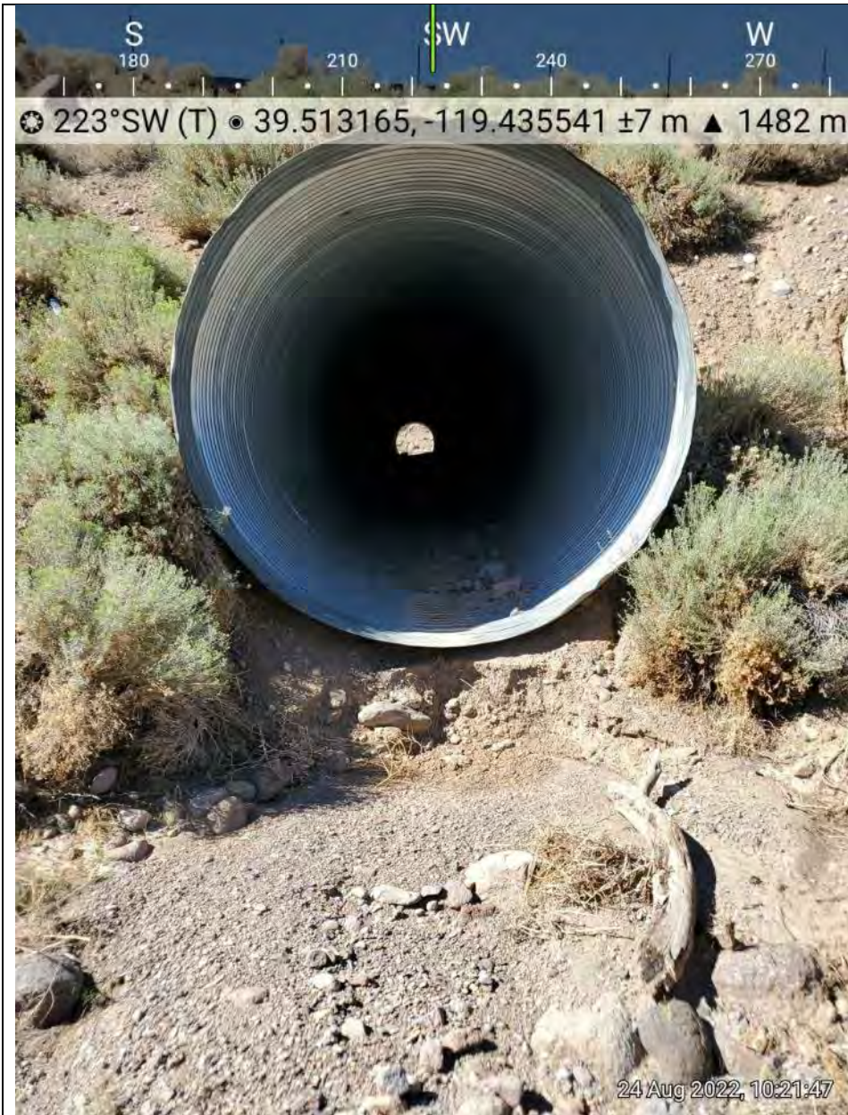
Photo 5. Culvert outlets after crossing under the USA Parkway. This culvert is one towards the middle position appeared to have the most flow activity.
