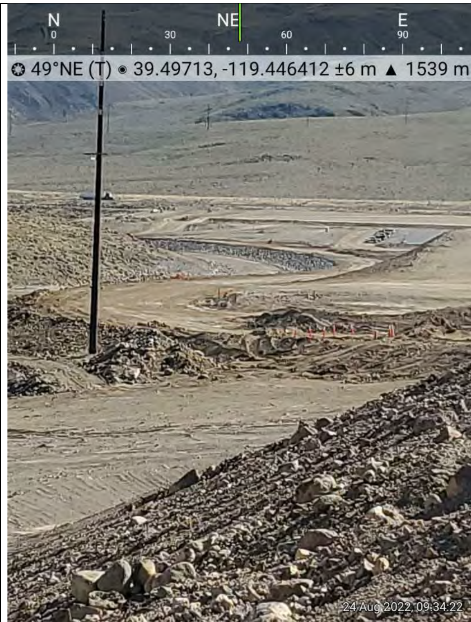
Photo 3. Looking down stream in AR 1, zoomed in beyond the non-disturbed area that was visible in the previous photo. This is the channel condition to the USA Parkway.
