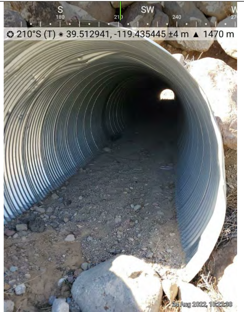
Photo 4. Culvert outlets after crossing under the USA Parkway. This culvert is the furthest to the left when looking towards the highway. Deposition does not appear to be bedload, but rather fill material from the slopes
