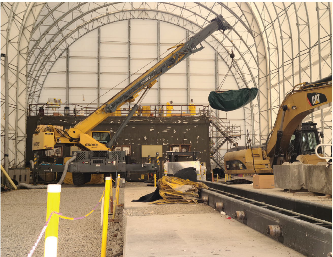
The roof of the hot cell was lifted to allow access into the structure
