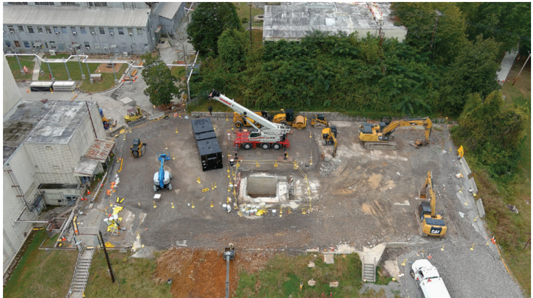
The reactor site after demolition (right) and the reactor structure being loaded into a special container for storage and shipment (below)
