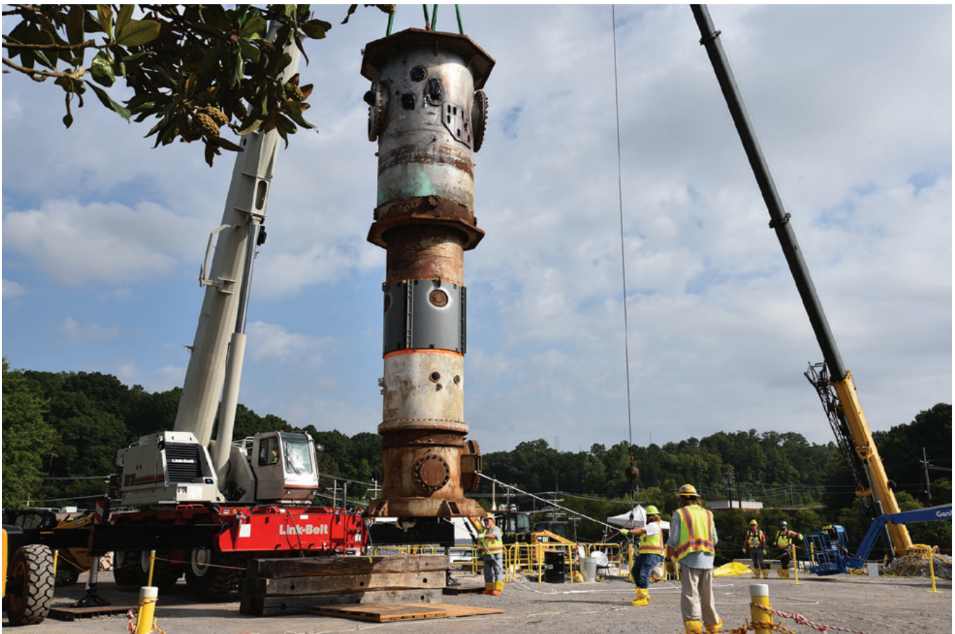
The 30-foot long reactor structure being lifted out of its housing to be placed in a storage container
