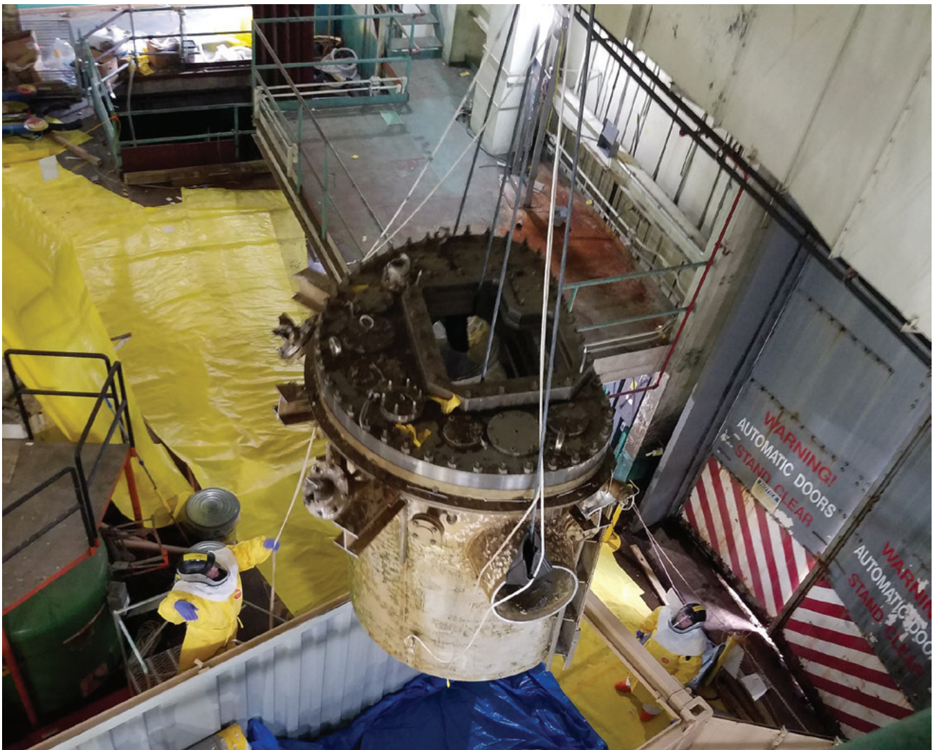
The top segment of the reactor structure was cut off, packaged, and removed from the building
