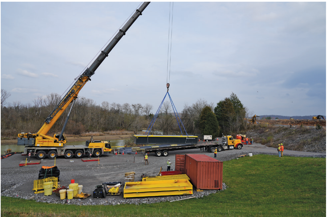
A crane is lifting a barge to be placed in the water and used to remediate the EU-19 mudflat
