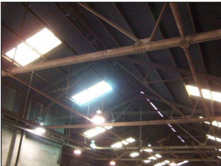
Roof system where supplemental limits were applied at the Aliquippa site (September 2005).
