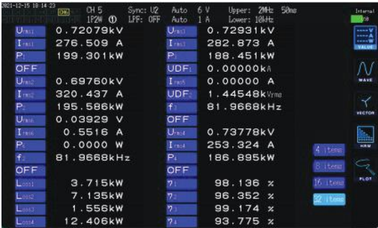
Figure II.3.3.6. Power analyzer reading for operation of 200 kW DWPT system at 186.6 kW output operation at 93.7 % efficiency.
