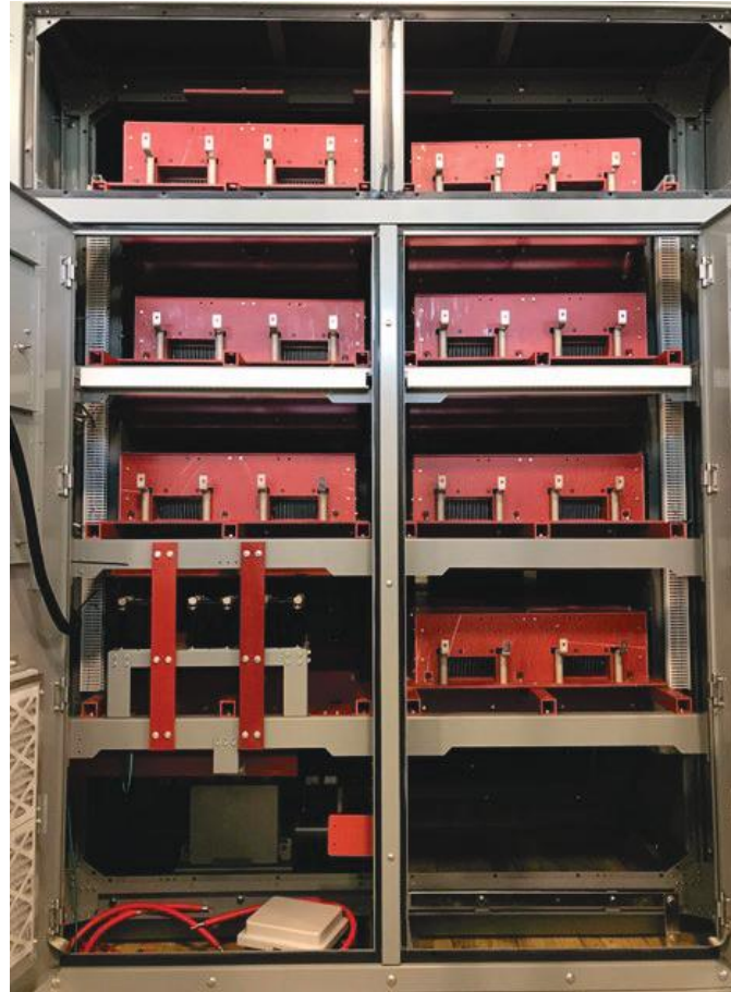
Figure II.1.8.6 DC – DC modules fitted inside the cabinet.
