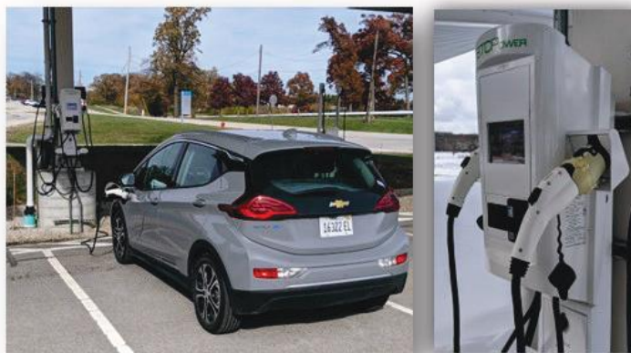
Figure II.4.2.3 Mk II SCA deployment at ANL Smart Energy Plaza.
