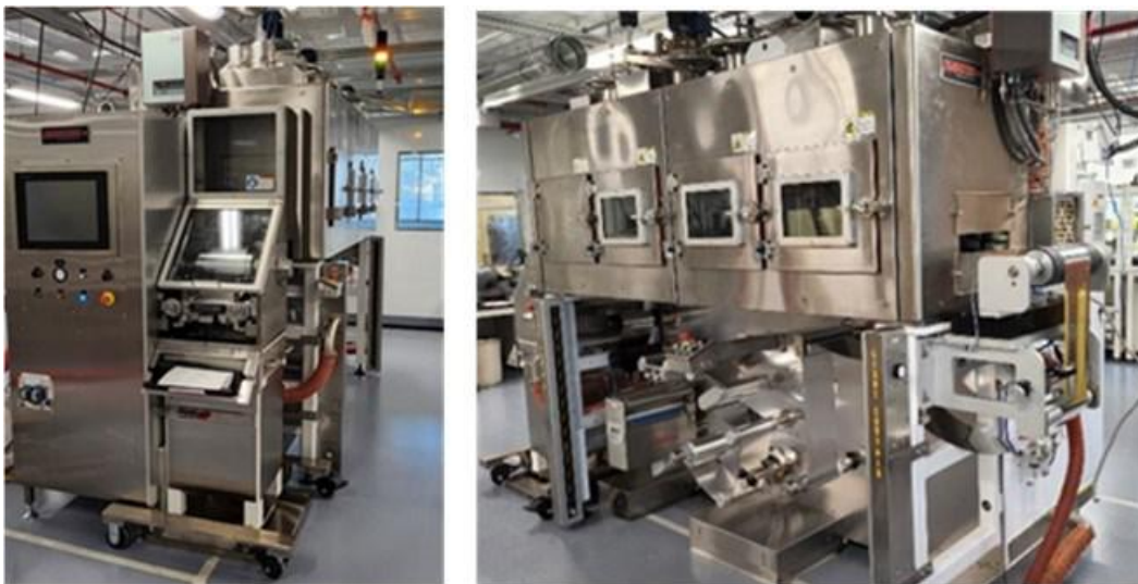
Figure VI.5.1 Images of the multifunctional coater installed in the CAMP Facility's dry room.
