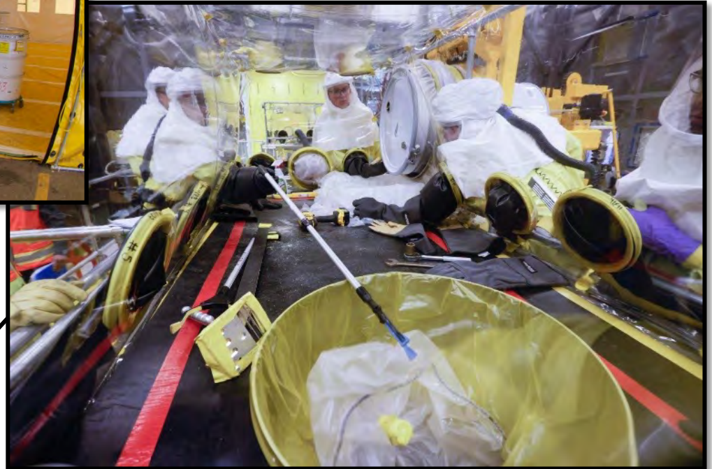
Mock-up of Dome 231 Glovebag Drill and Drain to Process Drums Not Compliant for WIPP
