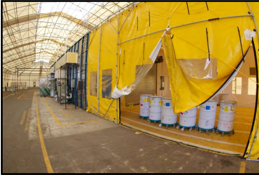
Drum Processing Area at PermaCon Inside Dome 231
