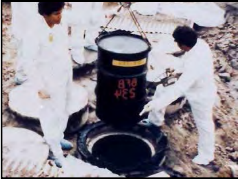
Arrays Have the Capacity to Hold Two 30-Gallon Drums Stacked One Above the Other
