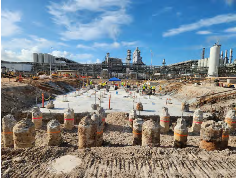
Photo 3: Area 310R18 Pile Bushing (OSBL South)
