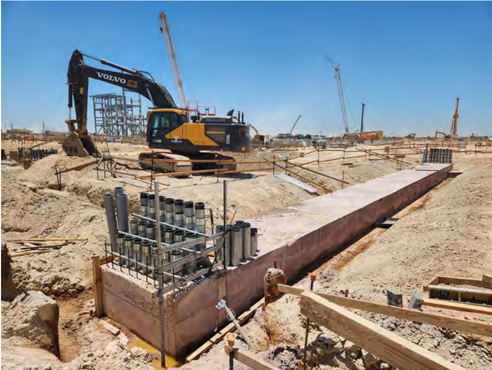
Photo 3: Electrical Ductbank at Liquefaction Substation (Train 1)
