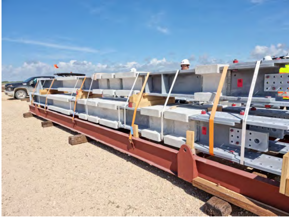
Photo 3: Fireproofed Steel on site
