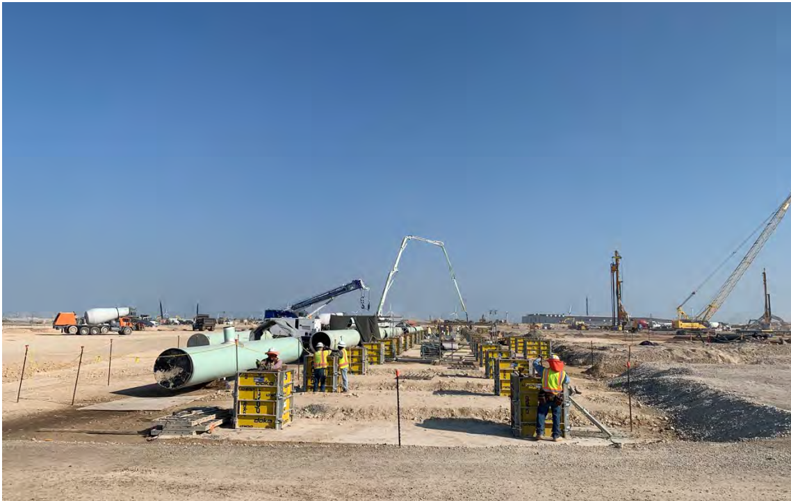
Photo 4: Preparation for piperack foundation pedestals work and 48-inch feed gas line (OSBL West)
