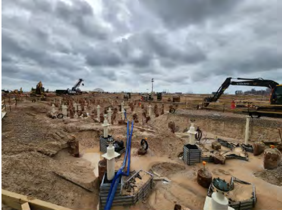
Photo 3: Train 1 Underground Amine Pipe
