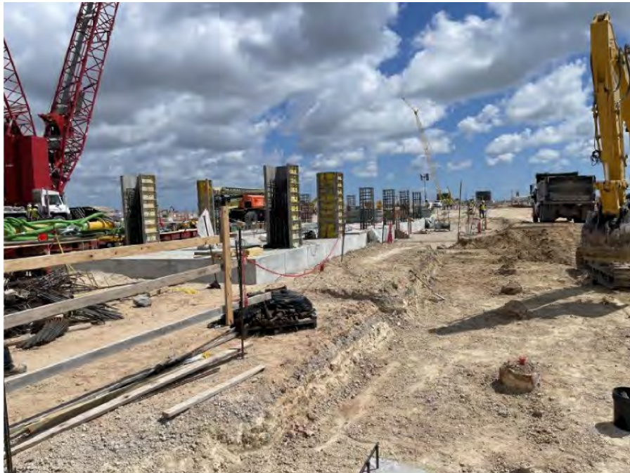
Photo 2: 311G01 Utility Substation Pedestals (Train 1)
