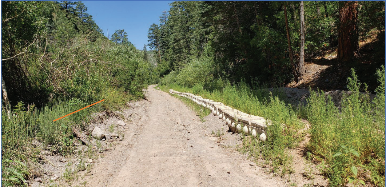
Photo 4. Road Washout and Temporary Pipeline Stabilization (orange line). This location will be filled with dredged material from the reservoir to raise the road up 3-4 feet above current elevation.
