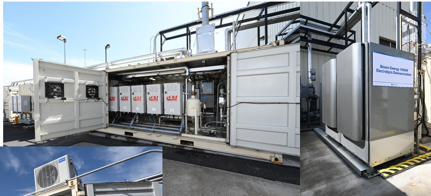
100 kW hydrogen+rectifiers outdoor with container
