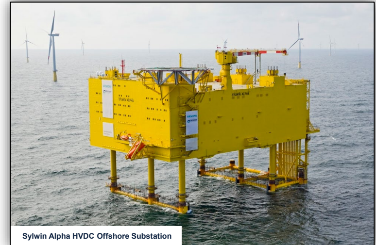
HVDC Converter Substation
