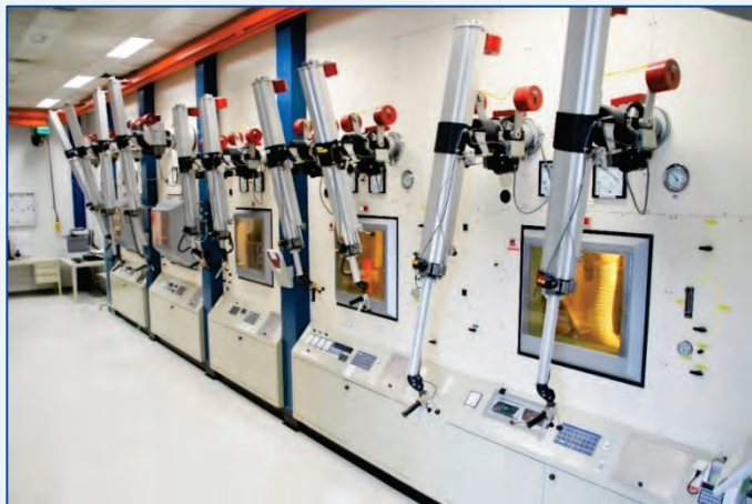
Hot cells used by the Dutch company Curium to produce Mo-99 using LEU targets. DOE/NNSA provided financial and technical support for Curium’s conversion from HEU to LEU in 2018.
