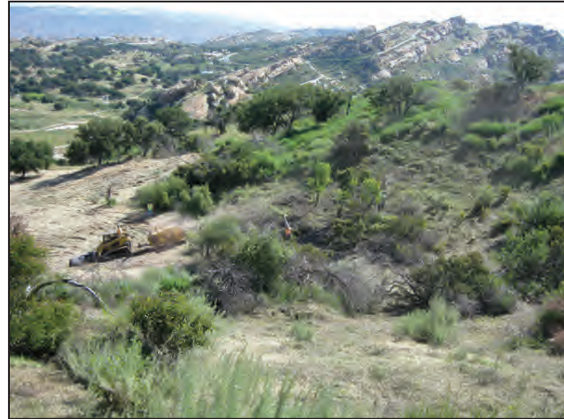
Plate 1B – Vegetation cutting activity in Subarea 5D South (SS-59) with active chipping. May 3, 2011.
