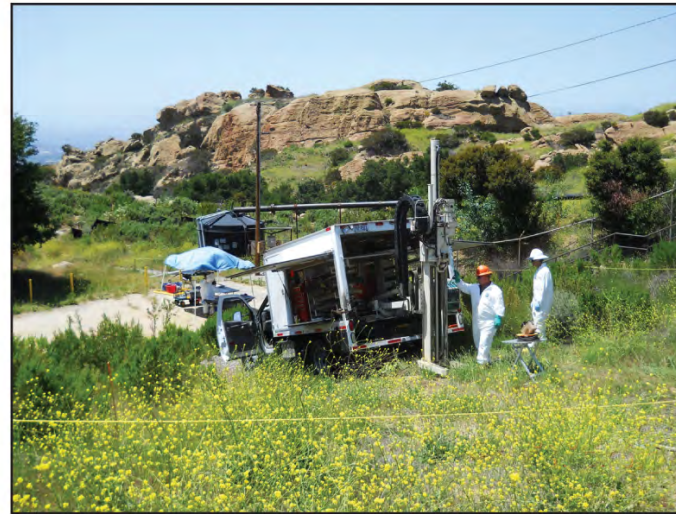
Photo 1B – Direct Push Technology rig in use in Subarea 7, operating within a roped area previously examined by a biological monitor and cleared for activities. Photo taken May 15, 2012.
