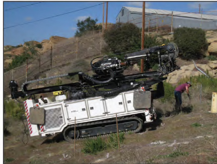
Plate 1D – Moving the subsurface soil sampling drill rig in Subarea 6 while avoiding a Santa Susana Tarplant that is identified by stakes to alert workers of its protected status. February 20, 2012.
