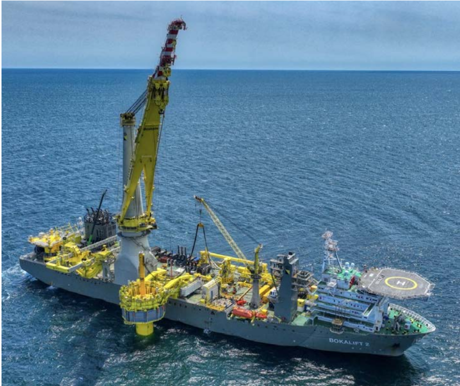
Installation of first monopile foundation at South Fork Wind Farm. Photo courtesy of South Fork/Boskalis
