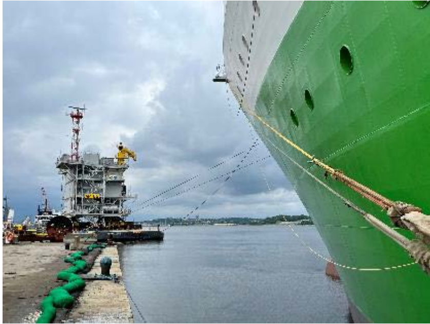
First offshore wind substation in the United States at Providence, Rhode Island, ready for installation at South Fork in June 2023. Photo courtesy of South Fork Wind Farm
