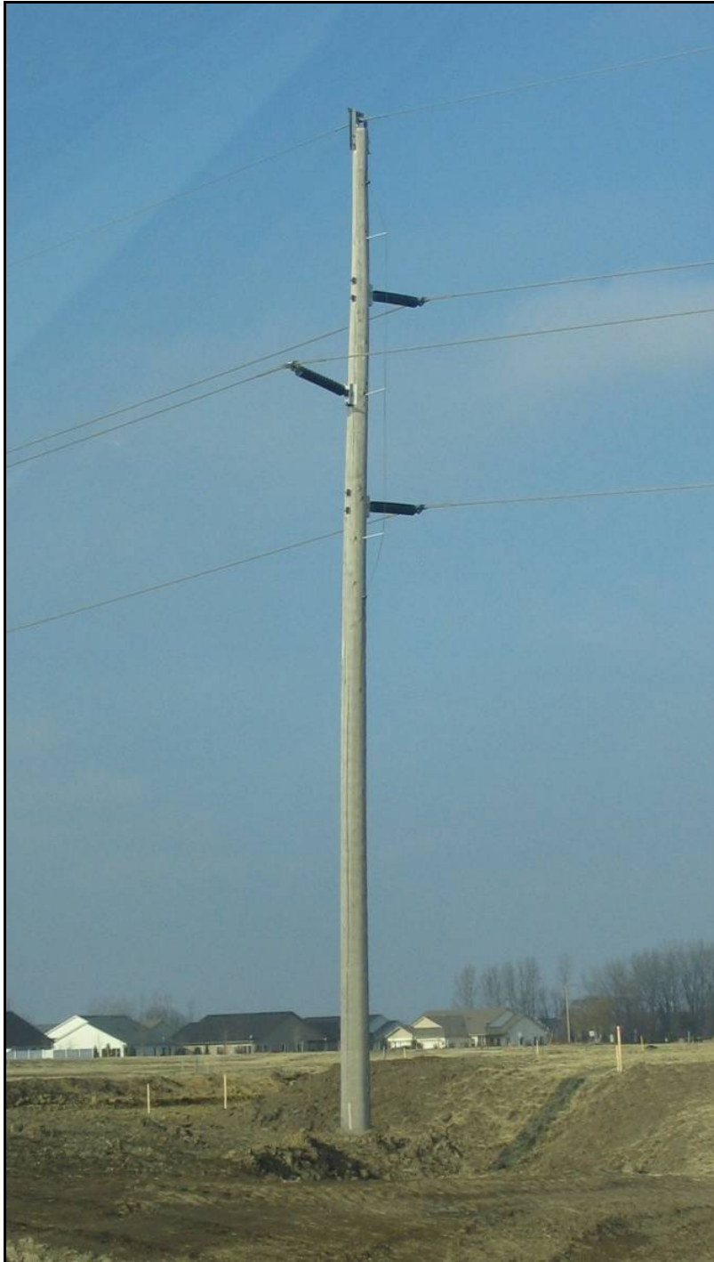
FIGURE 2.3-1 STANDARD SINGLE POLE 115-KV STRUCTURE
