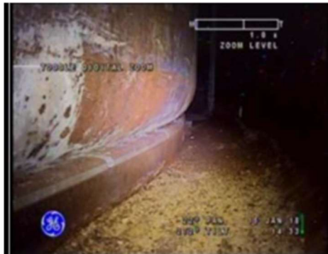
Tank AY-101 Annulus Floor Showing Debris
