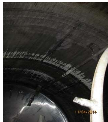
Secondary Process Tank Interior
