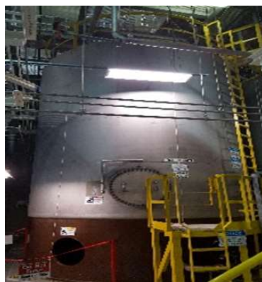
Secondary Waste Process Tank
