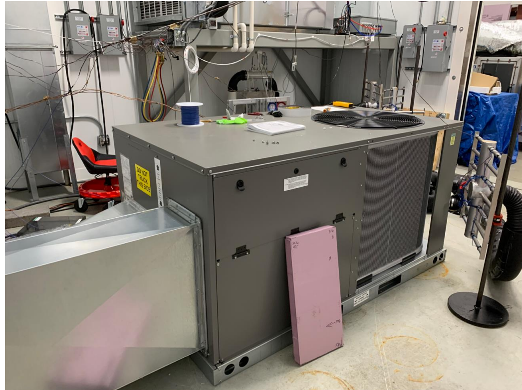
Commercial Roof-top Unit Used for Charge Prediction Validation
