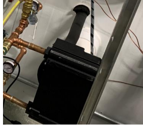
Compact brazed plate HX (in a plastic box, vented to outdoor via a PVC pipe)
