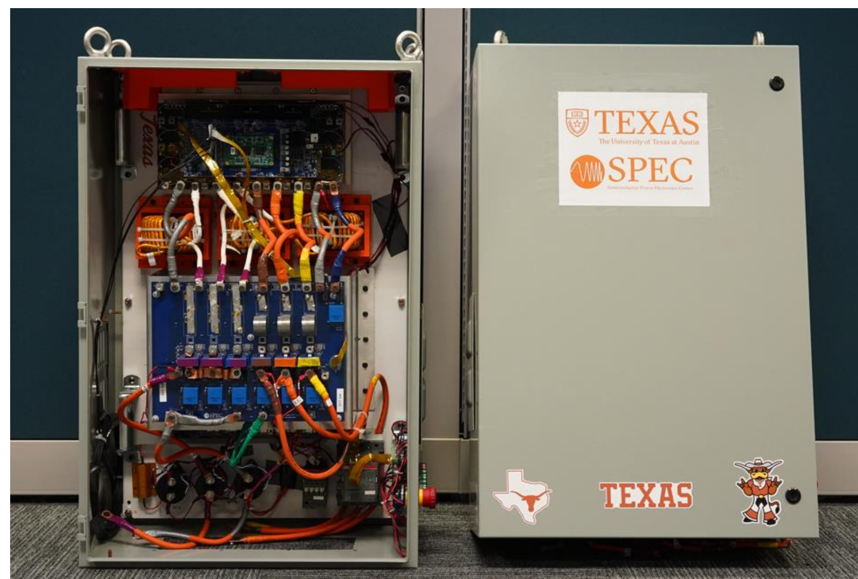
Fig. 2. 75kVA SiC Intelligent Power Stage (IPS)
