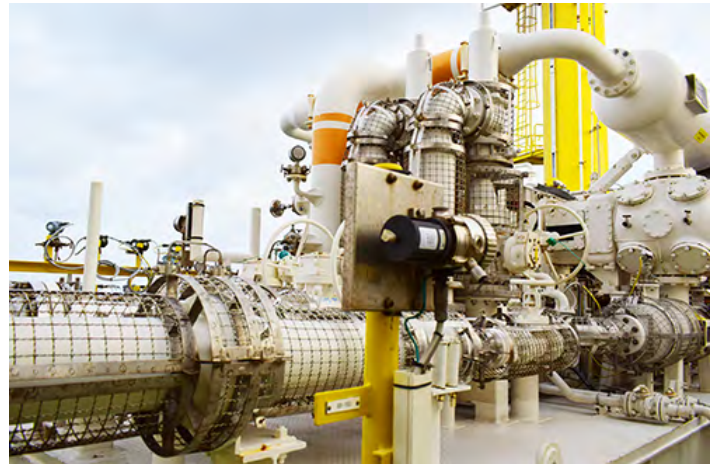
A gas detector provides a warning if a gas leak occurs.
