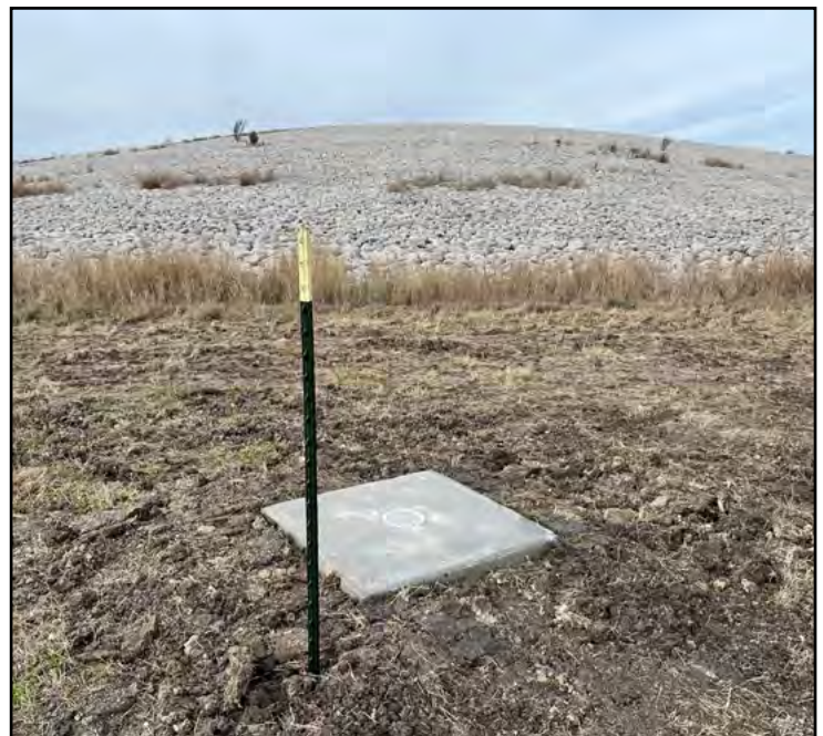
The finished product after concrete was poured to securely anchor a quality-control monument.
