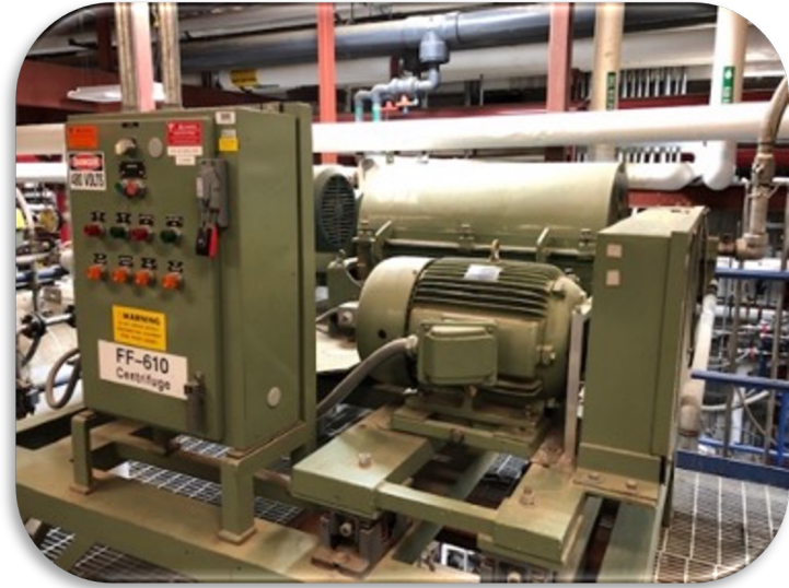
Pilot Plant Decanter
