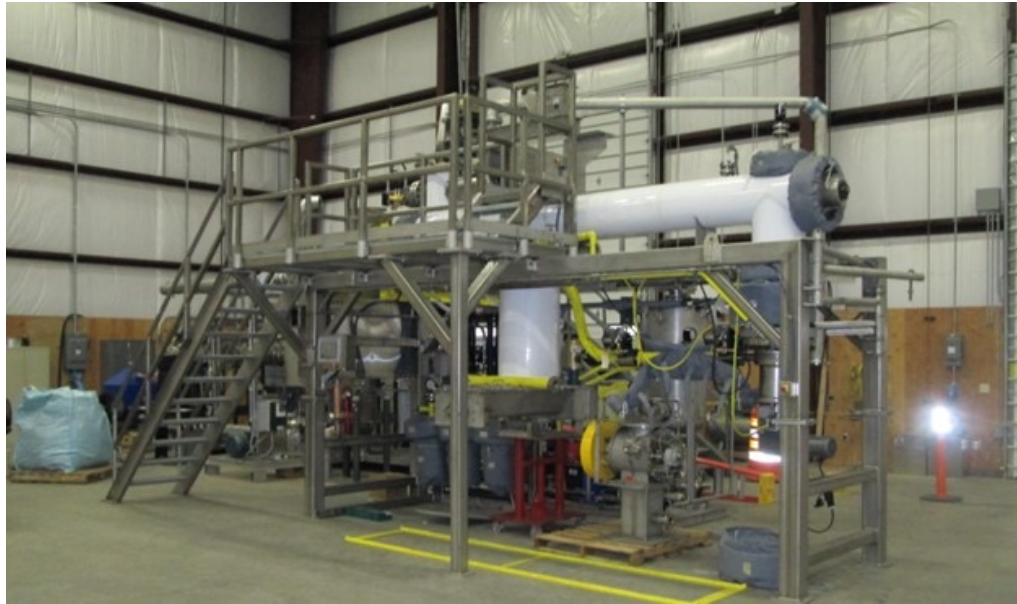
INL chemical preprocessing system (CPS)
