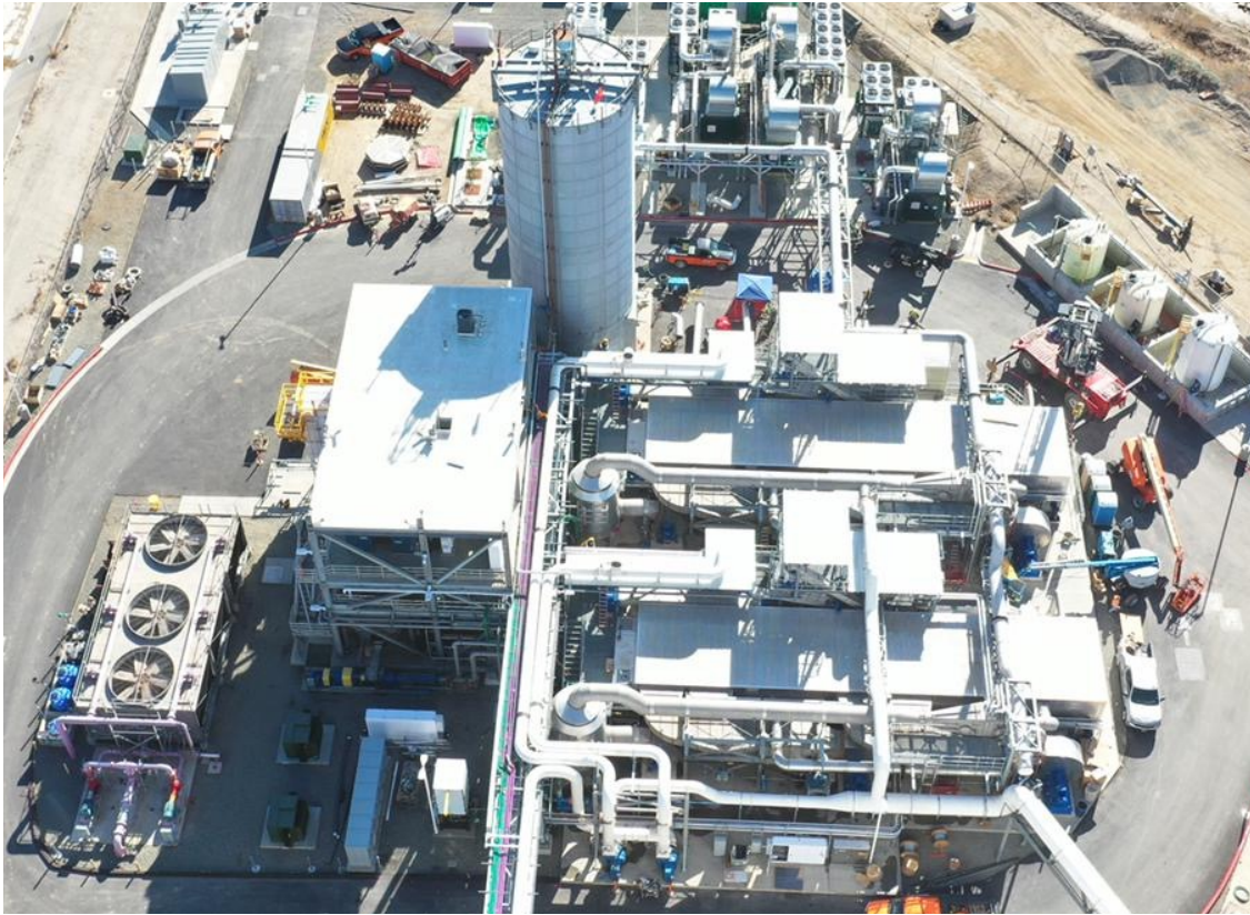
300 WTPD biosolids dryers currently installed and operating
