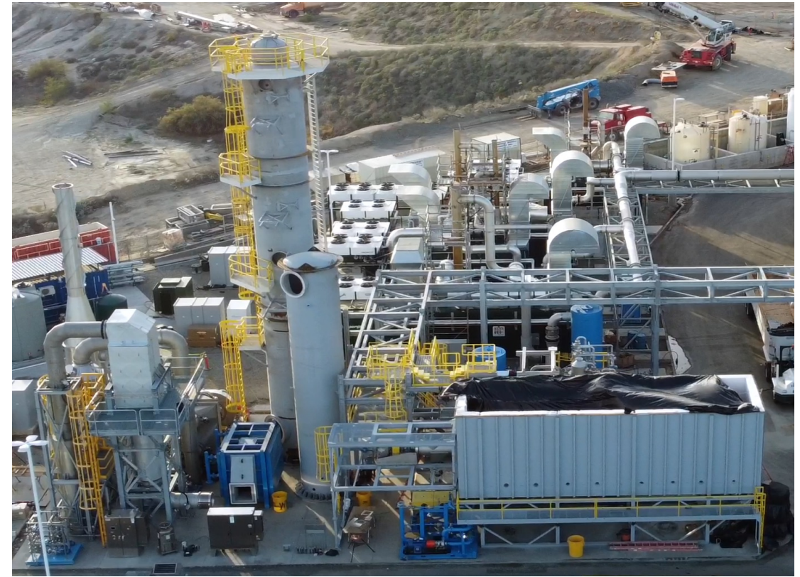
Pyrolysis Installation as of Dec 2022
