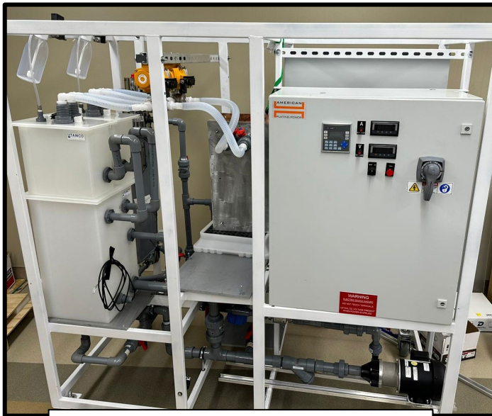
Pilot-scale NH 3 electrolysis skid
