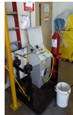
Biogas compression and filling unit (BRC FuelMaker).
