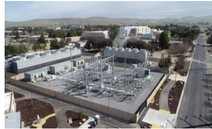
Upgraded cooling and electrical capabilities upon the completion of ECFM at LLNL
