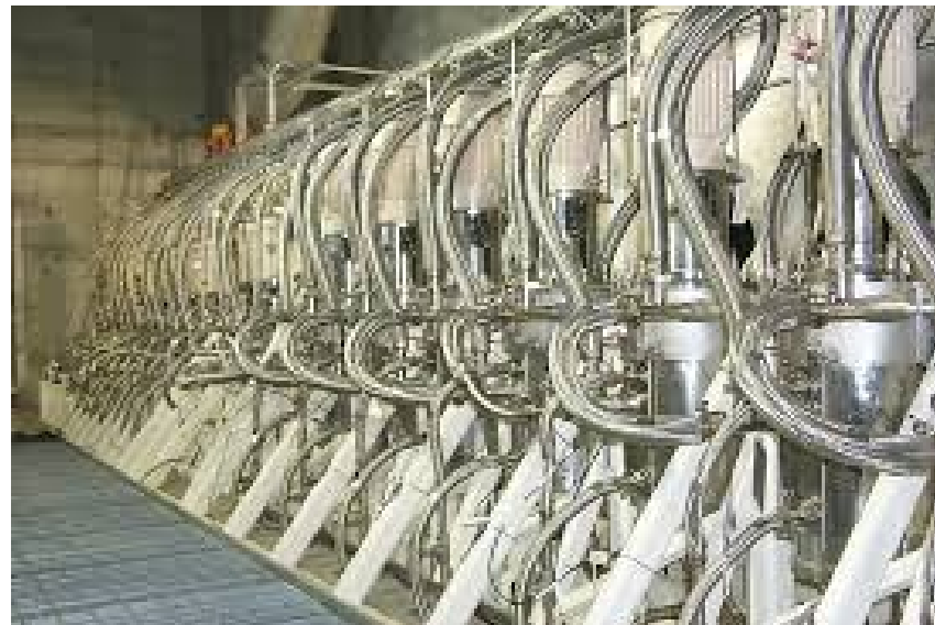
Contactors at MCU for mixing waste and solvent
