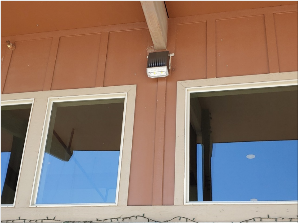
New Outside LED Lights
