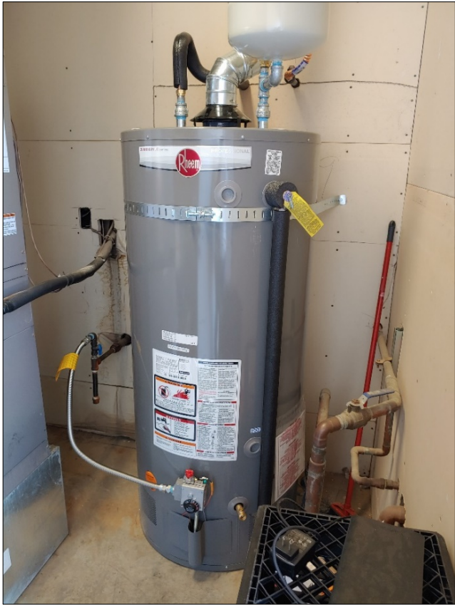
New Energy Efficient Propane Hot Water Heater
