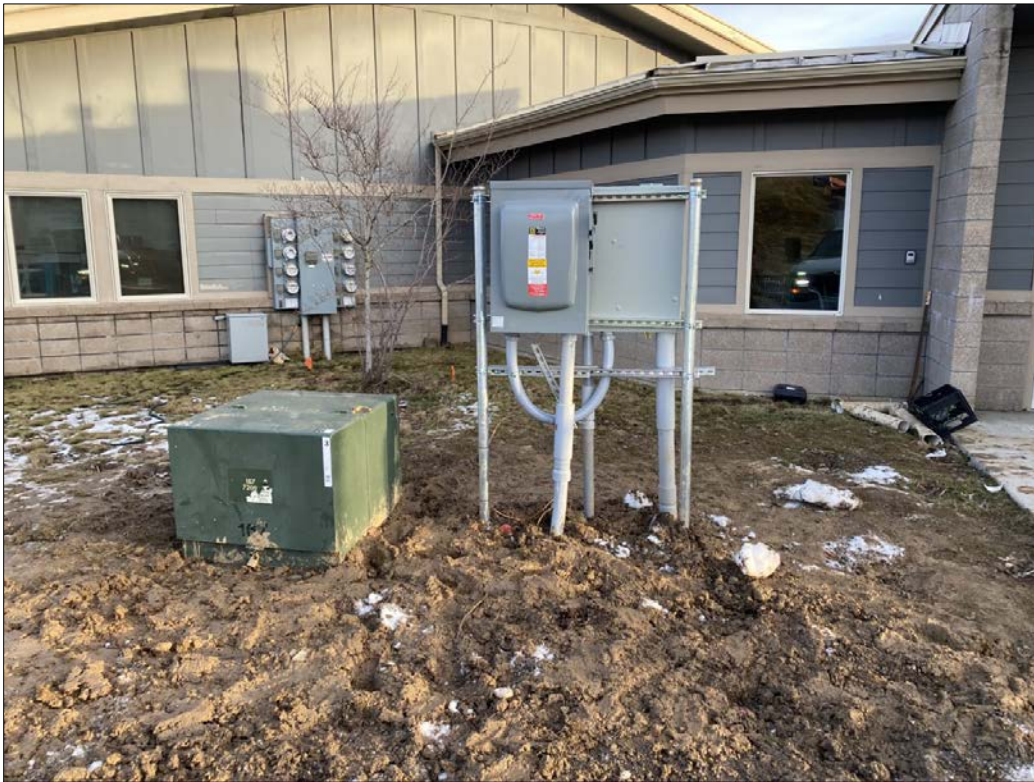
New Electrical Meter
