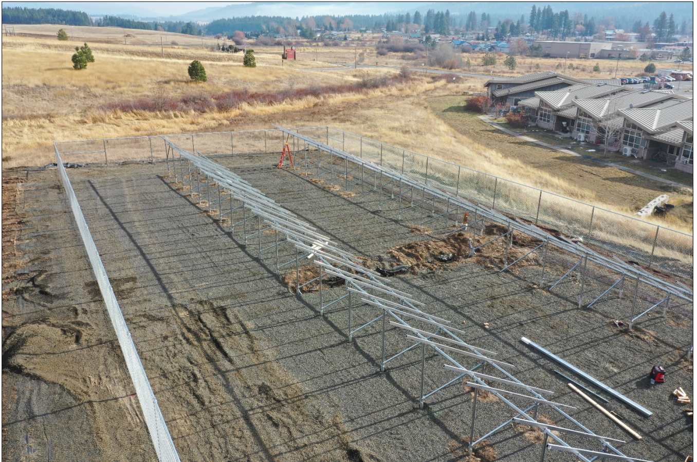
Fencing and Racking for Solar PV System
