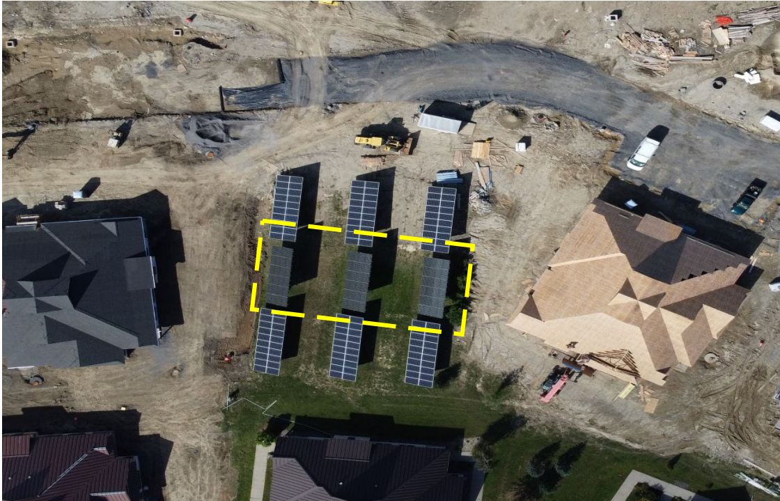
New Solar Arrays for Onsite Solar (net metering)
