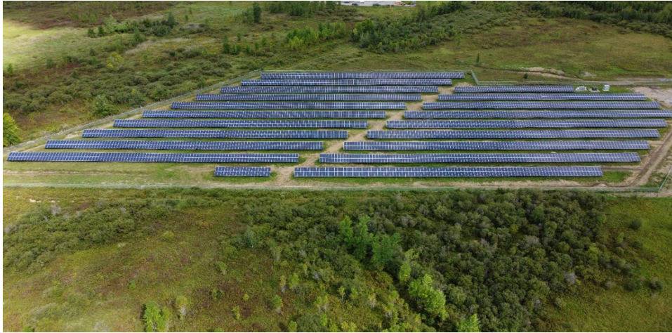
AHA 617 Kw Solar Farm Site as of September 2021
