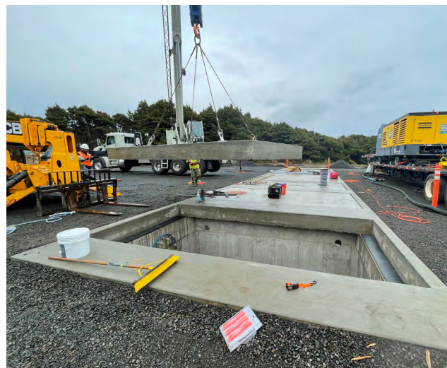
The PacWave underground cable vault is nearly completed with an opening showing where workers will be able to access subsea and terrestrial cables.
