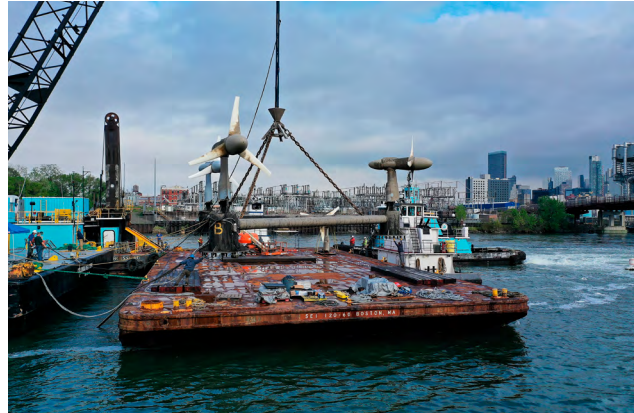
Verdant Power's deployment of its tidal power turbine represents an application of the TC 114 62600-200: Electricity producing tidal energy converters – Power performance assessment. Image from Drone Altitude
