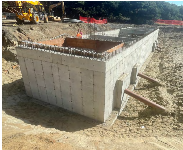
At the Driftwood Beach State Recreation Site near Newport, Oregon, the PacWave project team installed a 74-by-17-by-10-foot underground cable vault, where subsea cables will transition to terrestrial cables.
