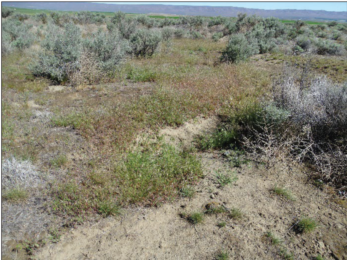
Figure 3. Sinkholes and Subsidence Areas at Nike Missile Launch Site H-83-L (WIDS 600-13)
