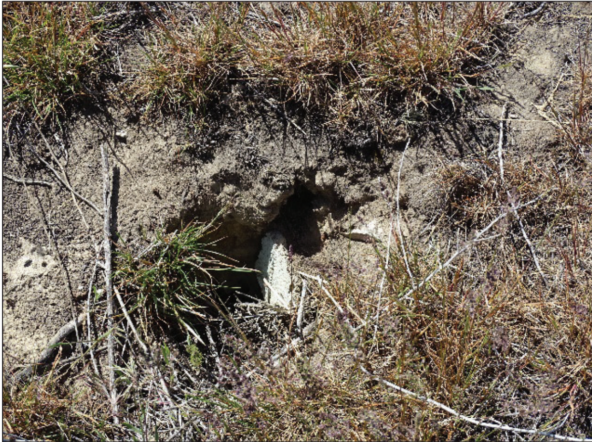
Figure 2. Sinkholes and Subsidence Areas at Nike Missile Launch Site H-06-L (WIDS 600-9)
