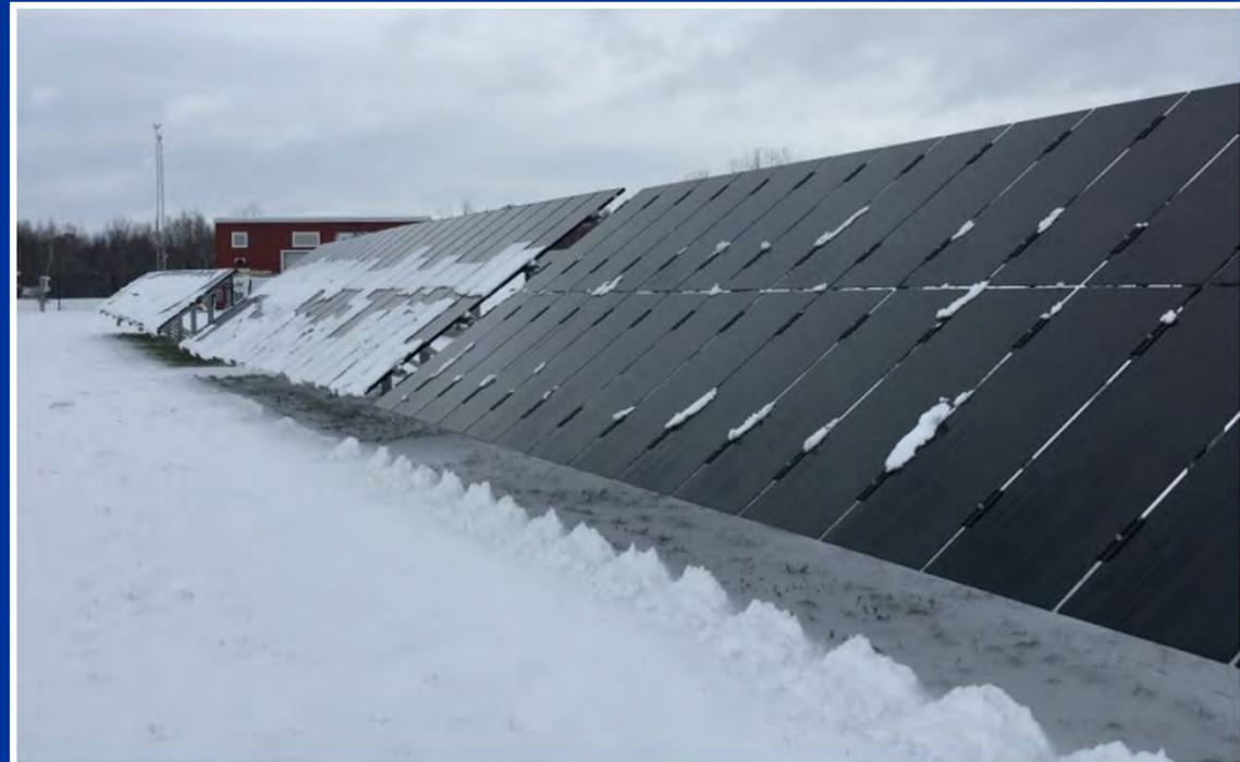
At the Regional Test Center in Williston, Vermont, researchers are examining how framed (in the background) and frameless (in the foreground) solar photovoltaic modules handle snowy conditions. | Photo Courtesy: Sandia National Laboratories
