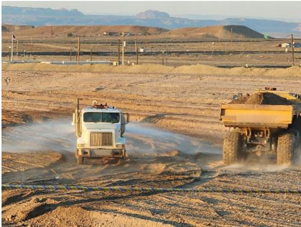
Photo 70. Dust Control September 2022
