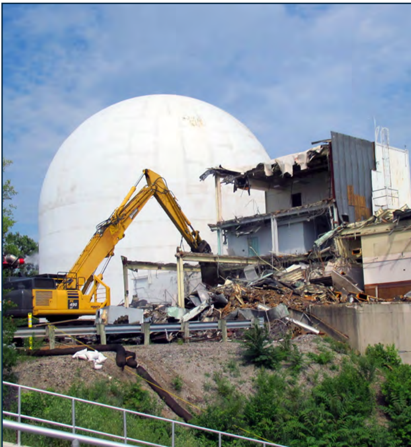
Auxiliary building in process of being removed at Piqua, Ohio, Decommissioned Reactor Site.
