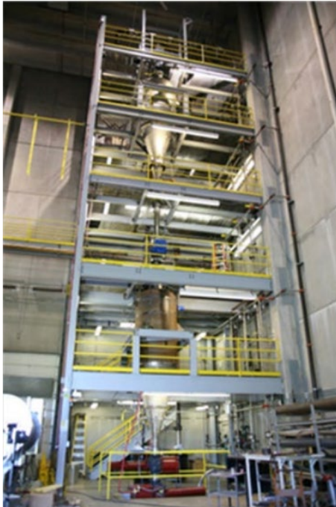
Test facility for the feed system
