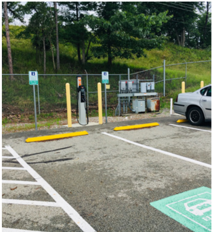
FIGURE 10 | Electric vehicle parking spaces and charging station at NETL
