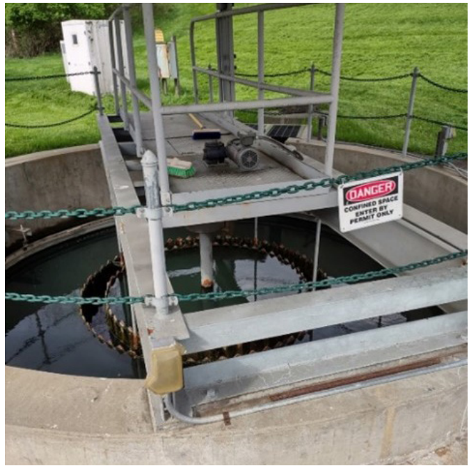
FIGURE 15 | Clarifier used for settling solids from industrial wastewater before discharge at NETL
