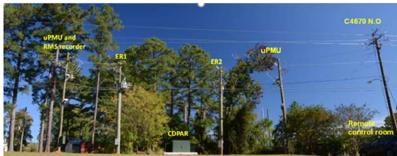
13 kV 1 MW Power Router Field Demo
