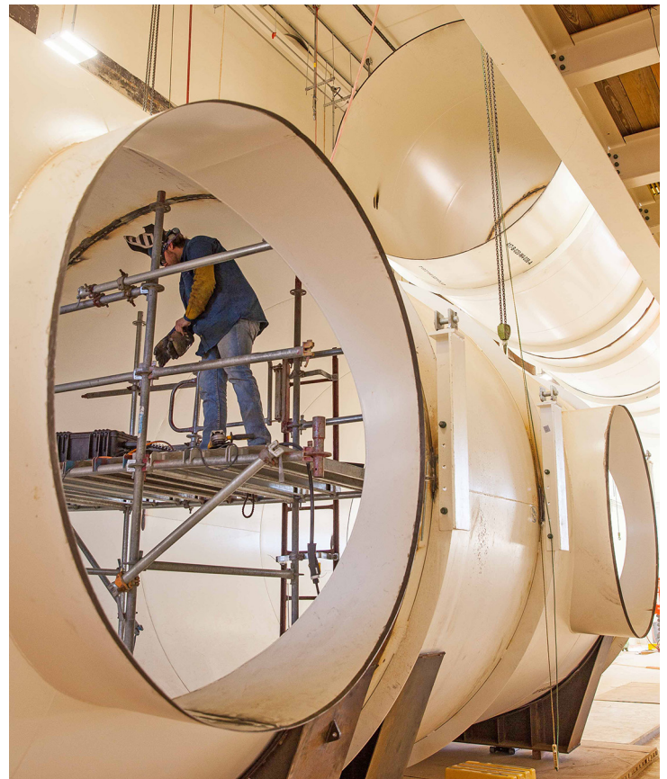
A worker inside the 14-foot ductwork of the SSCVS Project's Salt Reduction Building.
