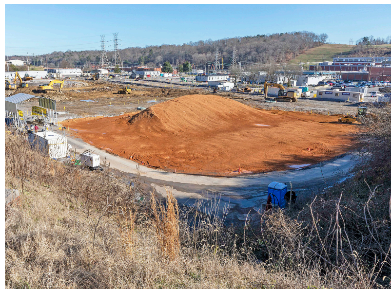
Soil is brought in to backfill the former Biology Complex area after slab removal.
