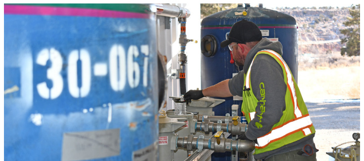
A crew member checks an Ion Exchange Unit where groundwater contaminated with hexavalent chromium is treated as part of the Interim Measures operations.
