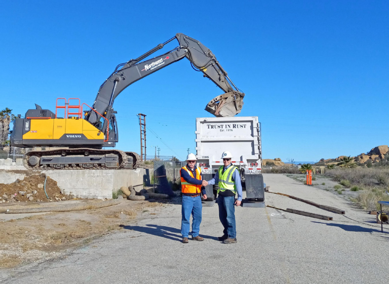
EM's federal project director at ETEC (right) shakes hands with a California Department of Toxic Substances Control Engineering Geologist as the last trucks of demolition waste safely left the site.
