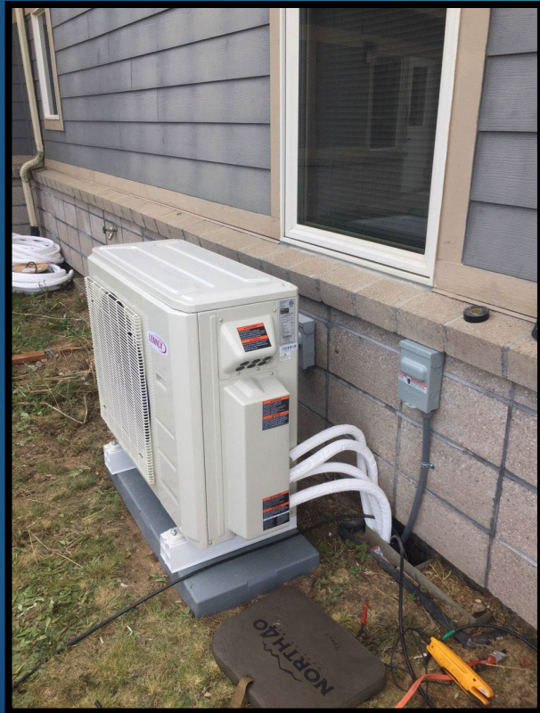
New Heat Pump – outside view
