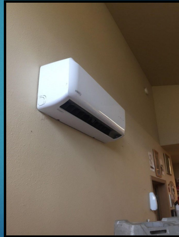
New Heat Pump – inside view
